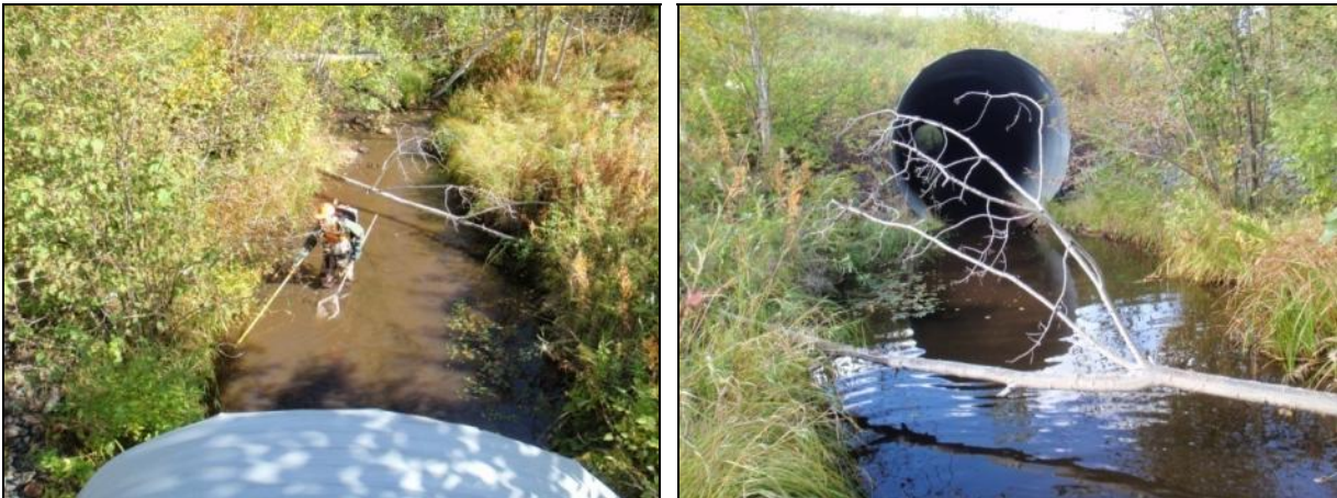
Figure 30. Muddy culvert pool below Site 17 on Whitewood River.
