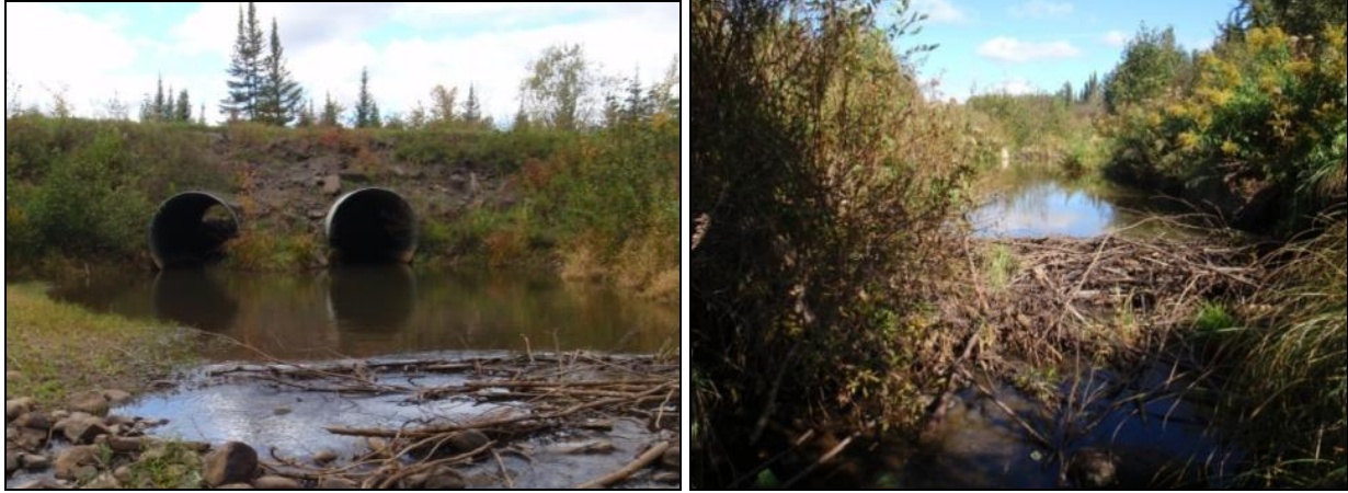
Figure 14 double culvert on Whitewood Creek at Hwy 590 (L) and Beaver dam on Rock Run Creek above Site 18 (R).
