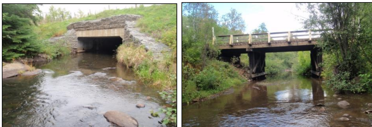
Figure 13. Box culvert on Cedar Cr. at Hwy 590 (L) and bridge over Whitewood Cr. at Smith Road (R).
