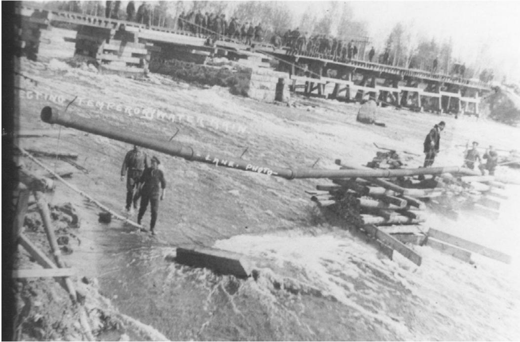
Erecting a temporary water main after the flood, June 1908. The civic railway bridge is in the background.
